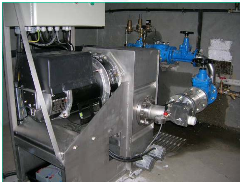
Turbine type PELTON 180 m - 5 l/s - 7 kW
