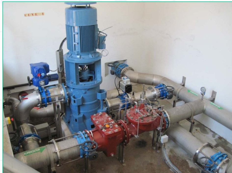
Turbine type Pompe Inversée 60 m - 70 l/s - 30 kW
